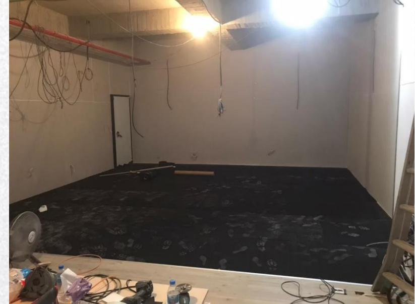
Rubber Anti-Vibration Pad (after construction)
