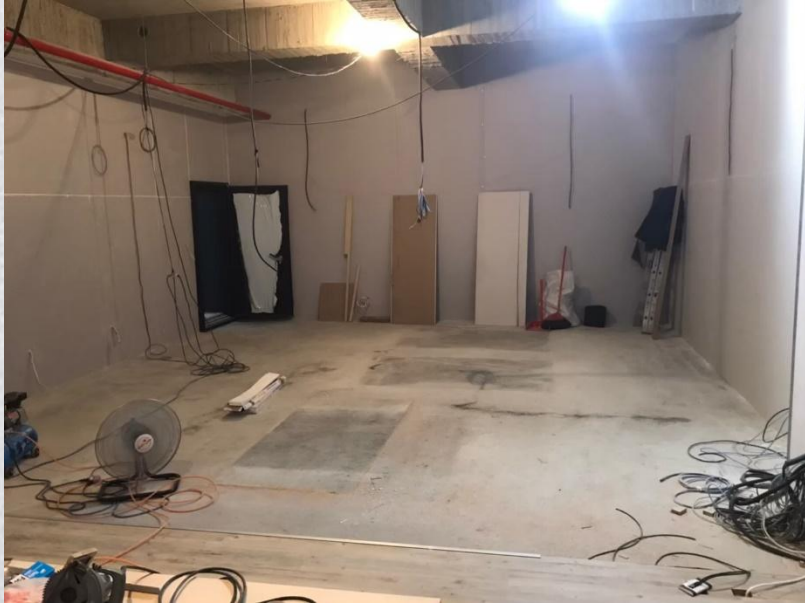
Rubber Anti-Vibration Pad (pre-construction)
