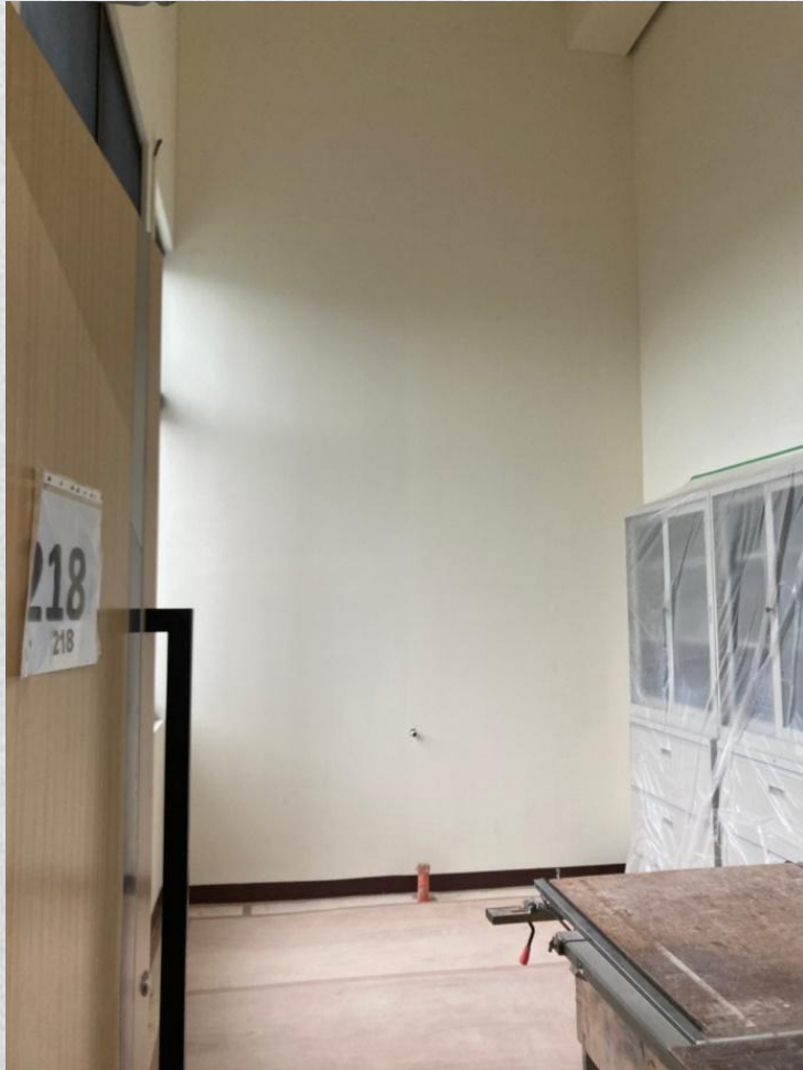
Sound Isolation blanket (pre-construction)
