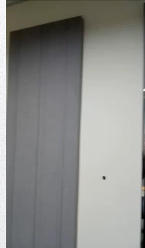
Downstairs received hits noise from the upper floors. Measurement: 60.3dB
