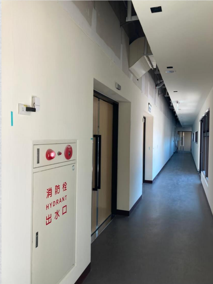
Sound Isolation blanket (pre-construction)
